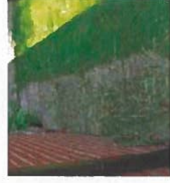
Poor Lot Grading
